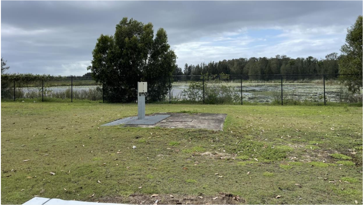
Photo 17 Sewer pump station and Basin 1 in background
